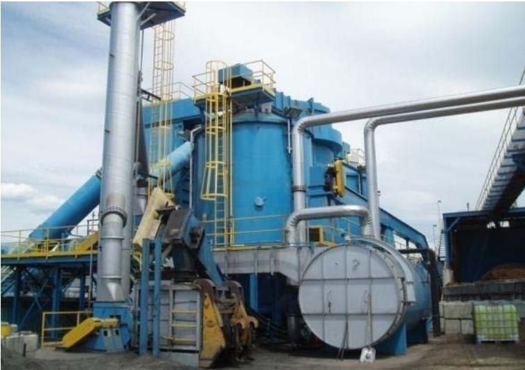
Nexterra Gasifiers and Boiler at Hefley Plywood, Tolko, BC (2006)
