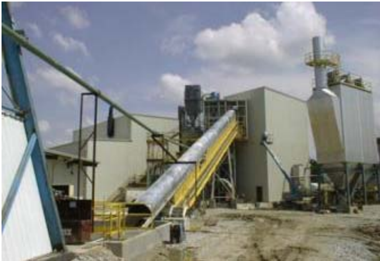
Energy Products of Idaho Gasifier at BFC Gas & Electric, IA (1998)
